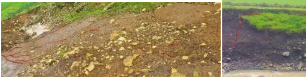
Pictures showing active cracks (red lines) on the banks of the river which is about to collapse
